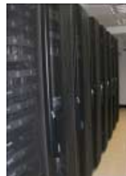
Techgate Data Centre
